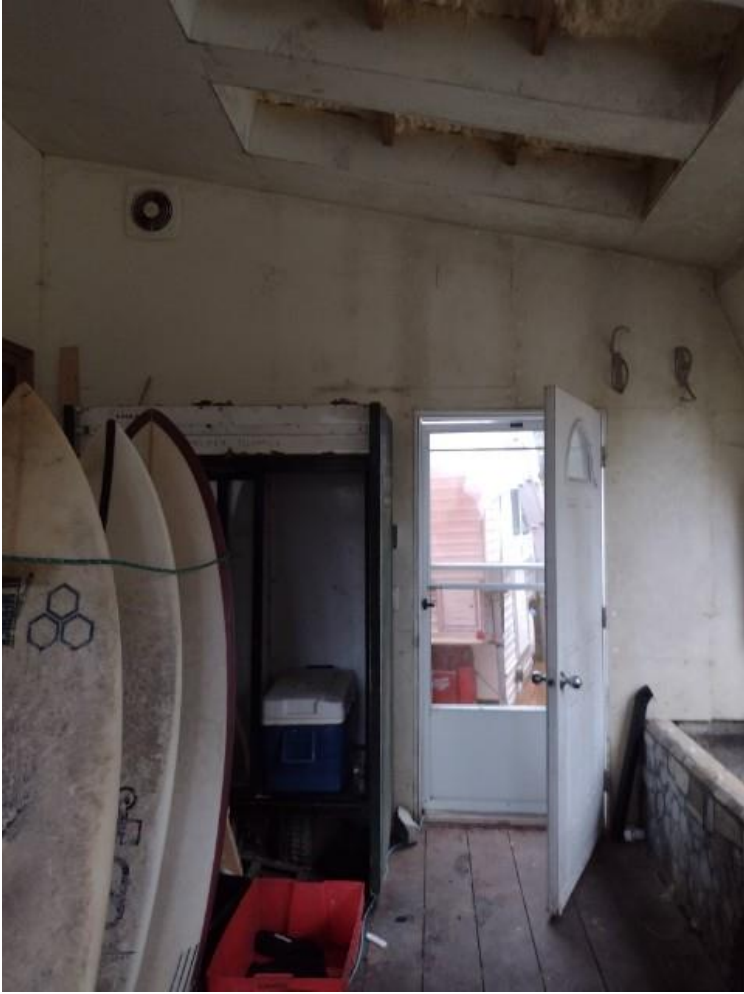
Atrium Interior: Moisture issues (mold, mildew) can be noted on walls and ceiling in atrium.
